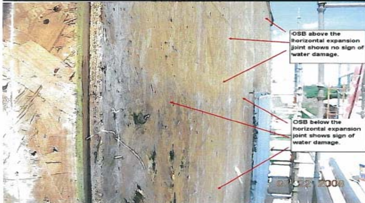
PHOTO # 8. Water damaged OSB along entire horizontal joint from NE corner to east master bedroom window.
