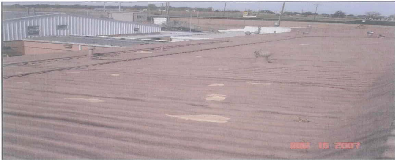
35. This photograph shows some of the repair attempts. The lighter colored areas are repairs made between 2002 and 2006.
