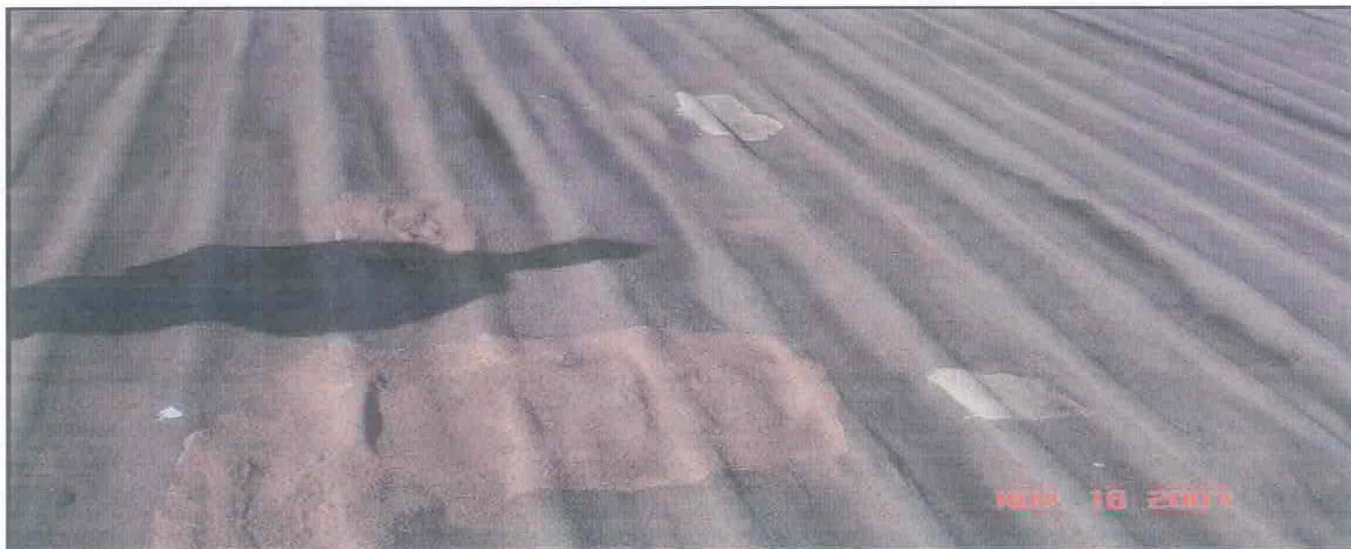
36. This photograph shows another area of repairs. The darker colored repairs were made in December 2006.
