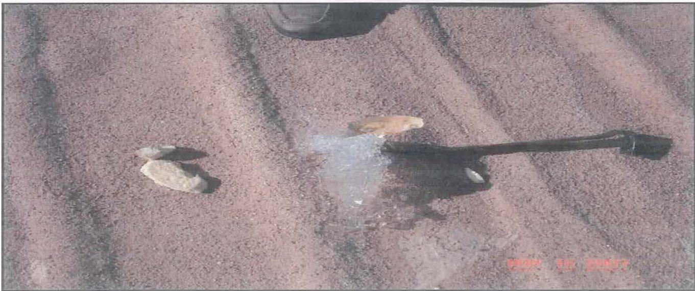
80. This photograph shows water shooting out of a big water blister.
